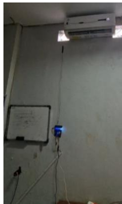
Fig. 2: Smart room site with sensor installation
